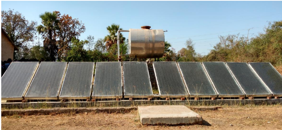
Solar water Heating System with capacity of 1000 LPD
