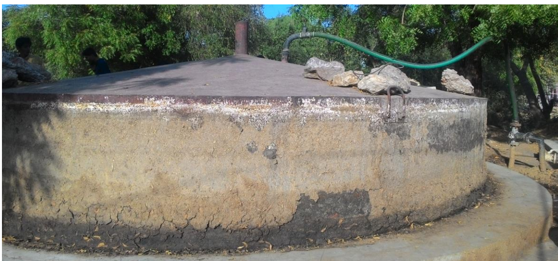
K.V.I.C Bio Gas Plant
