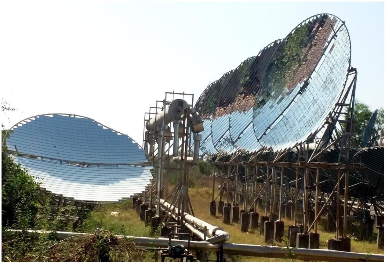
Parabolic Scheffler Dish (Total 100 Nos. of dish are installed)
