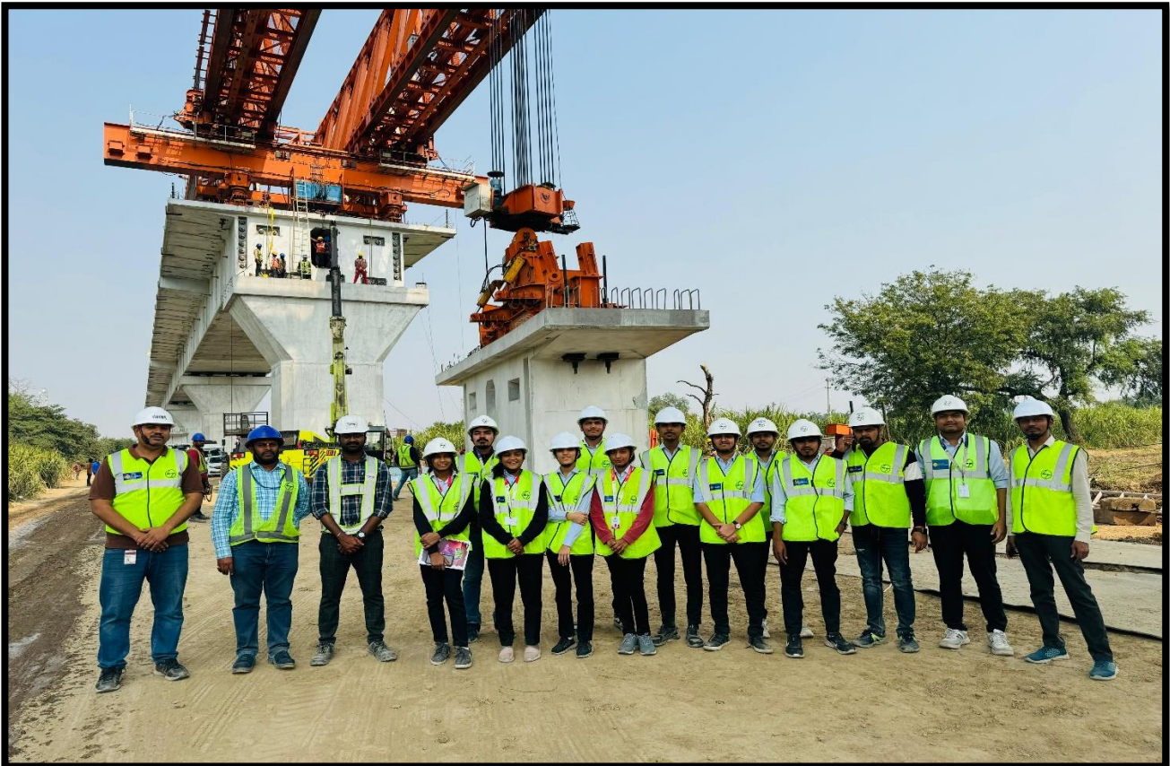
Group photo at Segmental casting yard site and Segmental spans erection site
